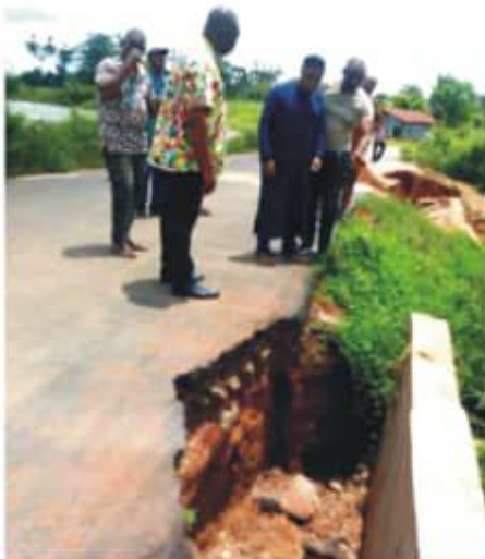
The ED at the Erosion Site near the Institute's Dam
