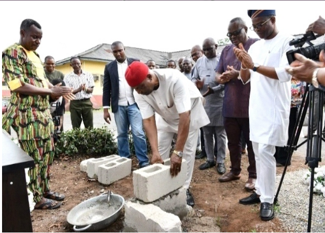
Laying of foundation for the 1000 capacity International Conference Centre during the Workshop
